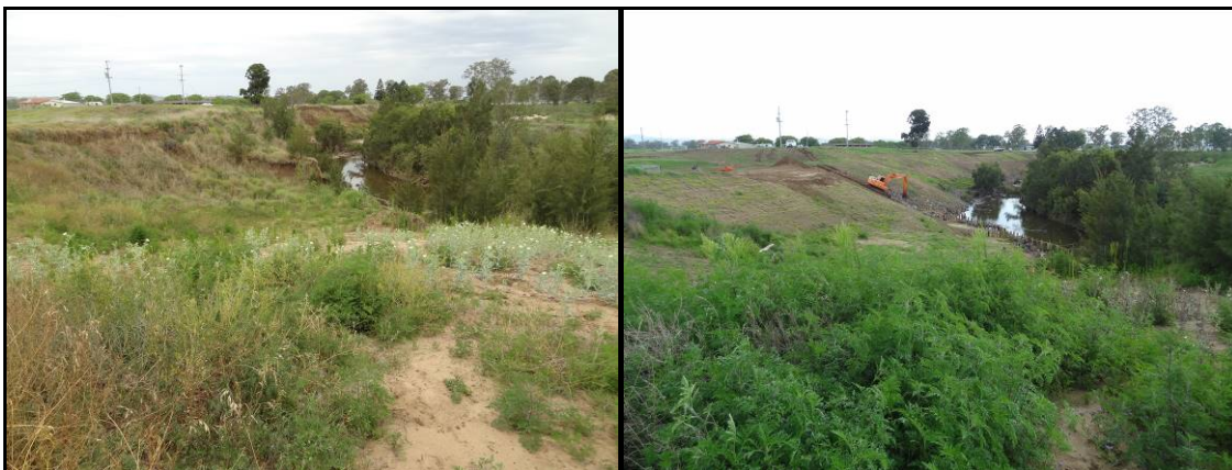
Figure 3: The larger Reach affected by fluvial scour – (a) prior to restoration; and (b) immediately post restoration earthworks
